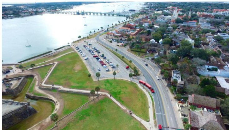
Duval Asphalt Products for their project on SR 5A (King St. and Avenida Menendez) in St. Augustine, FL in St. Johns County. Tonnage: 755
