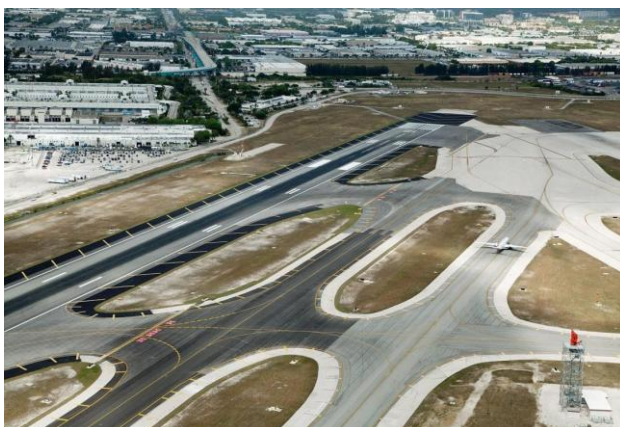
Community Asphalt Corporation for their project on MIA Runway 12-30 Pavement Rehabilitation in Miami-Dade County. Tonnage: 147,627
