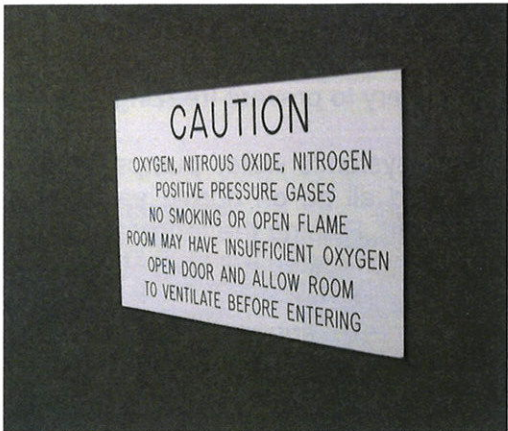
Figure 19. Equipment Room Wall Plate.
